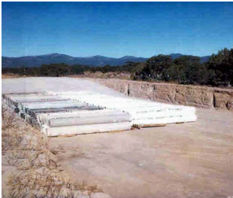
TA-54: 158 CMPs buried at the east end of Pit 29 above low-level radioactive waste
