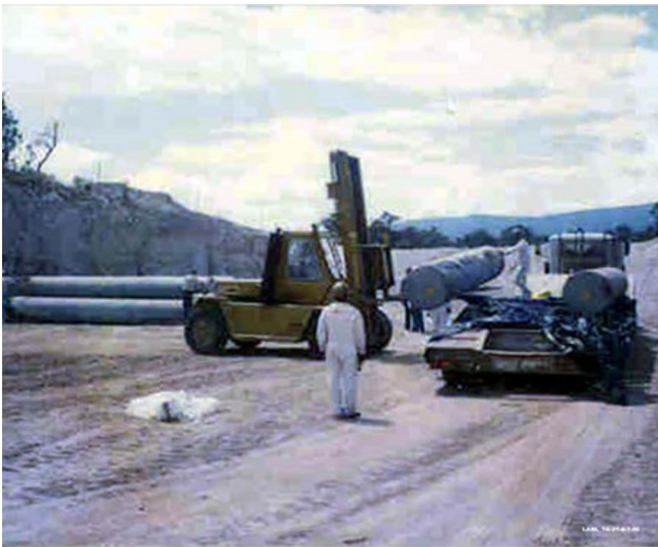
TA-21: 1986, CMPs were dug up, cleaned, decontaminated, wrapped in plastic & moved to TA-54
